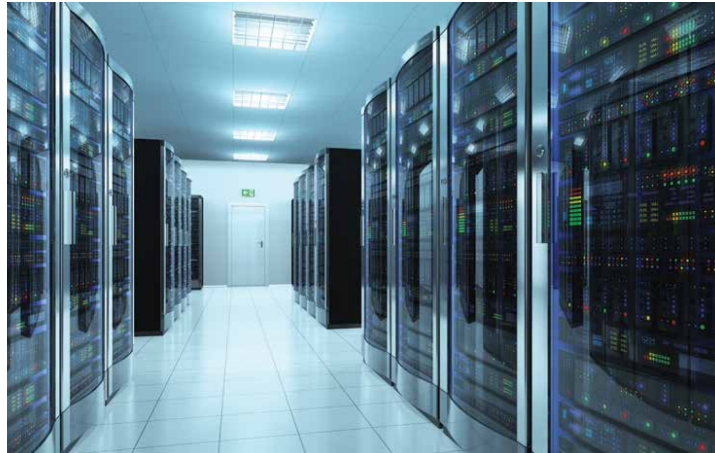
Server room, Vodafone España
